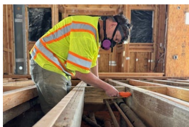
Hazardous building material field assessment
